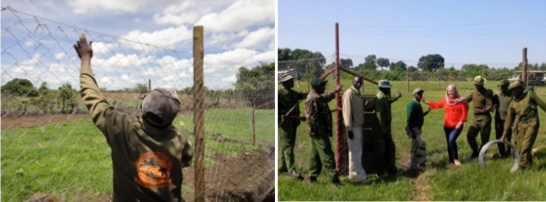
The AKTF carpenters finishing installation of the wire mesh on a new metal-corner boma (left), and Anne and the AKTF Team posing with a recently completed metal-corner boma (right)
